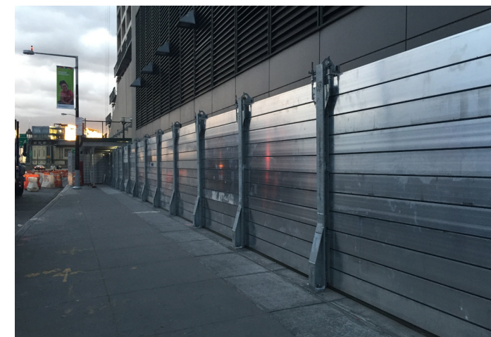
Example of dry floodproofing of a building in Lower Manhattan.
