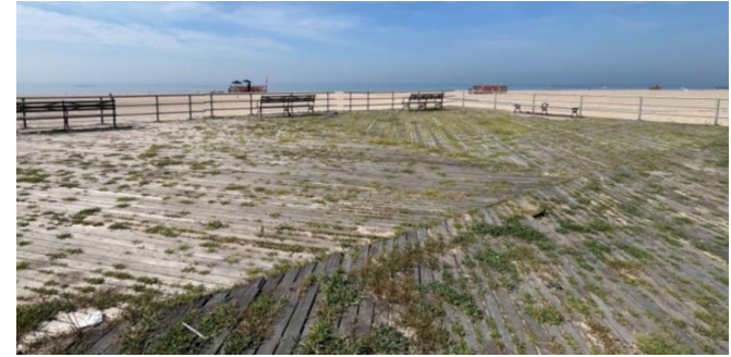
Rotting timber decking due to weeds, sand, and water
