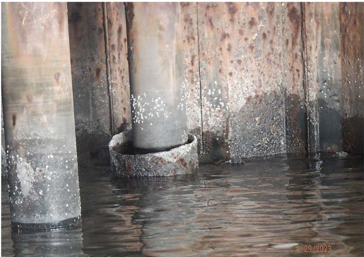
Photo 3.3-2: Example of a protective pile sleeve along the "E" row.
