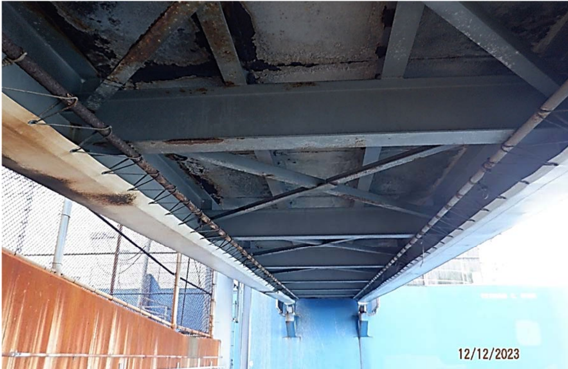
Photo 3.6-3: Overall view of the steel framing below the West Pedestrian Gangway A. Note the steel exhibits minor coating loss with corrosion at isolated locations on the floor beams and cross-braces.
