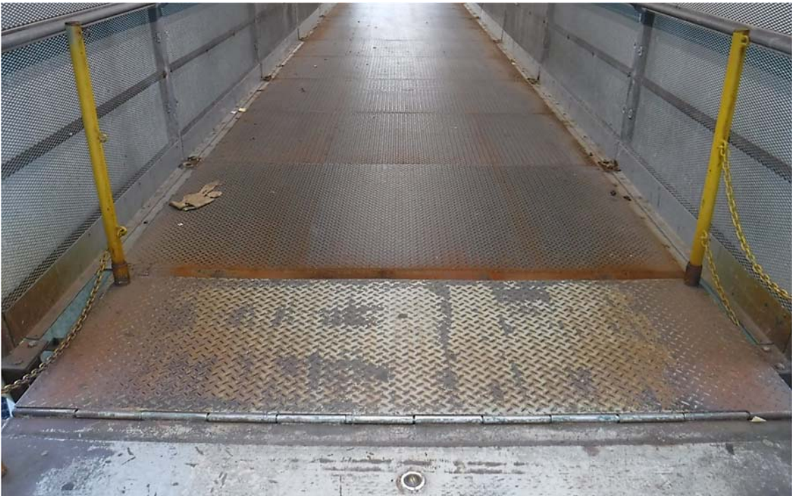
Photo 3.8-5: Interior view of the East Pedestrian Gangway C. Note the wear and minor surface corrosion at various locations and at the transition plate.
