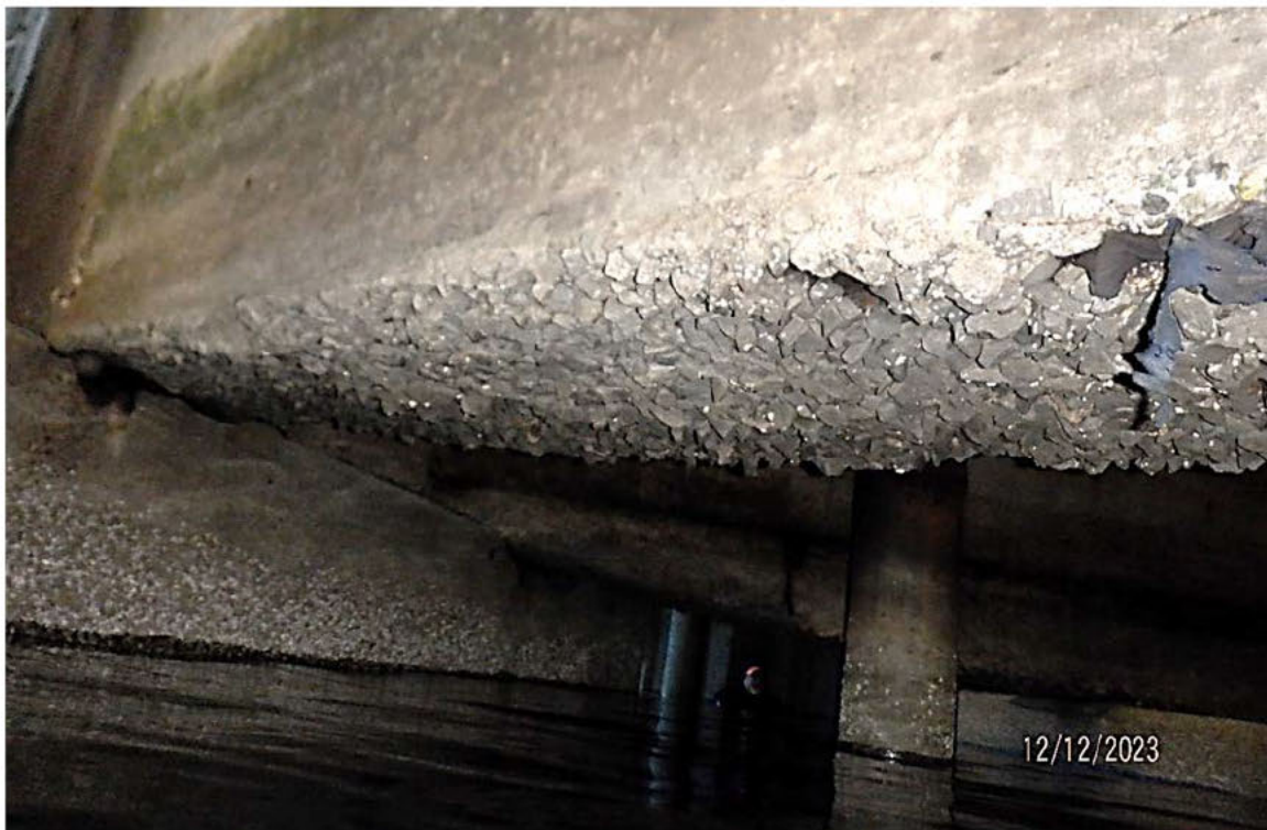
Photo 3.5-8: Typical condition of the strut underside illustrating gravel adhering to the underside of the concrete.
