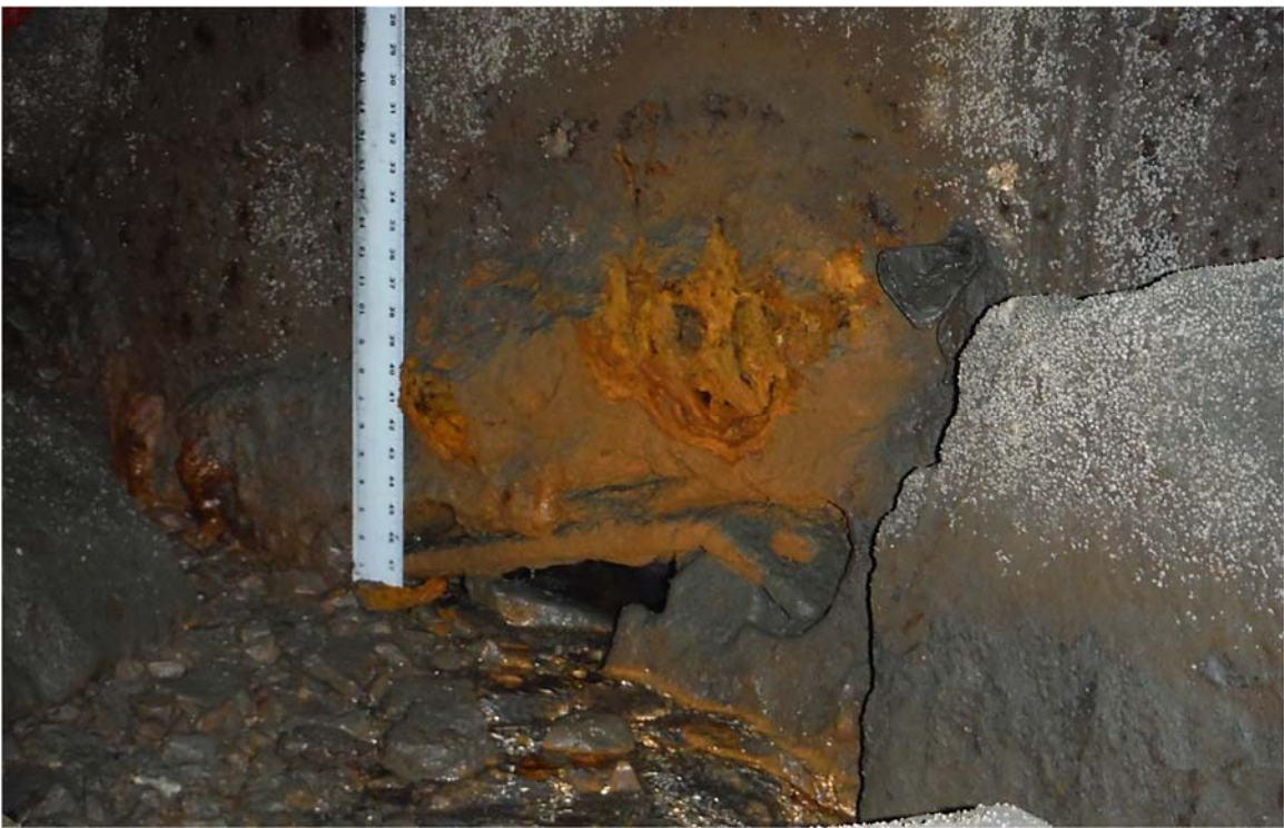
Photo 3.3-7: Severe localized corrosion and corrosion hole in steel plate below the west strut of the double-bit mooring arm. Note the void through the hole.
