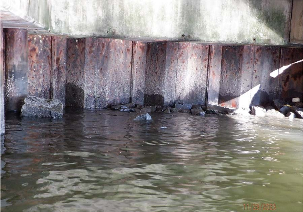
Photo 3.3-6: Typical coating loss and corrosion of the sheet pile cut-off wall in the splash zone.
