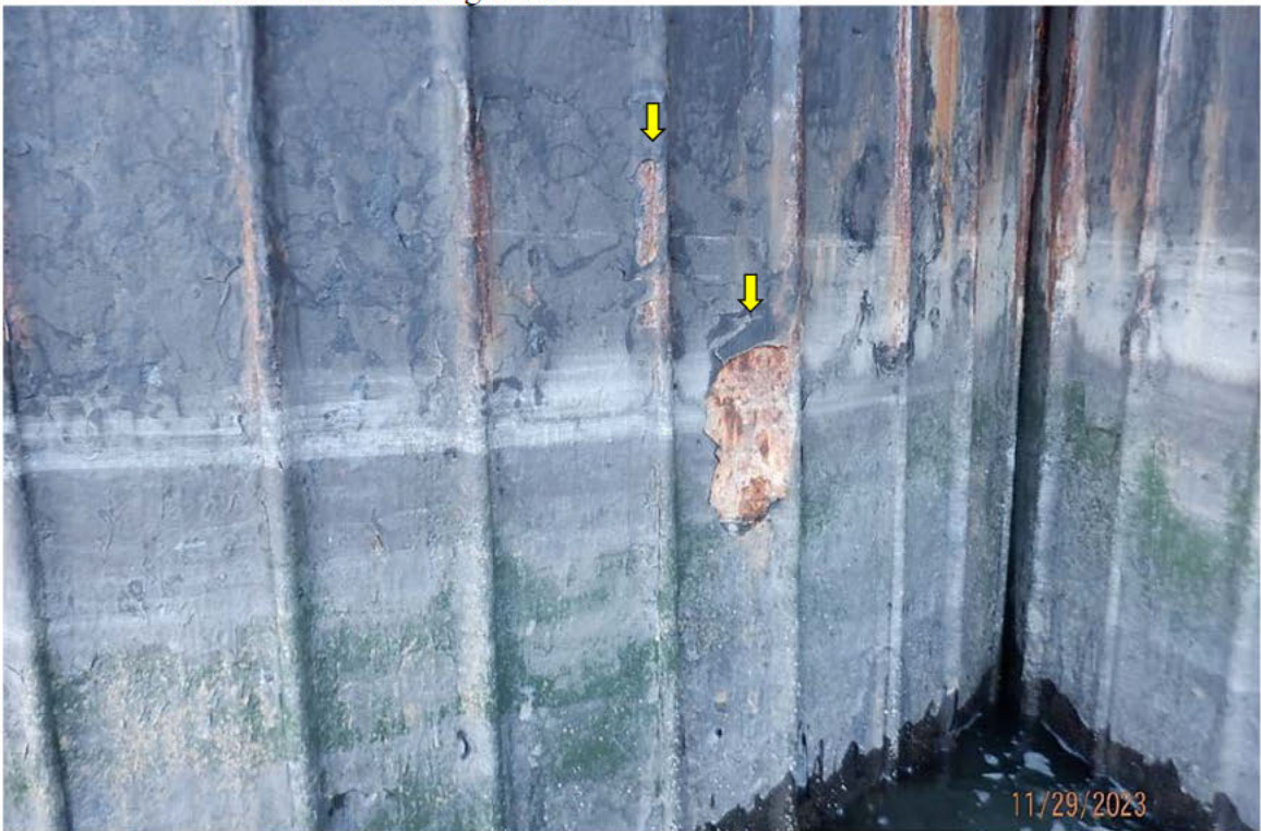
Photo 3.1-3: Example of coating failure in the tidal and splash zones above MHW. Note the interlocking joint knuckles typically exhibit coating failure.
