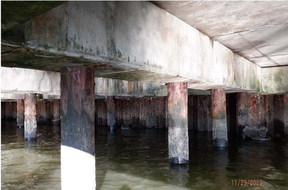
Photo 3.3-1: Typical condition of the steel pipe piles in the tidal and splash zones.
