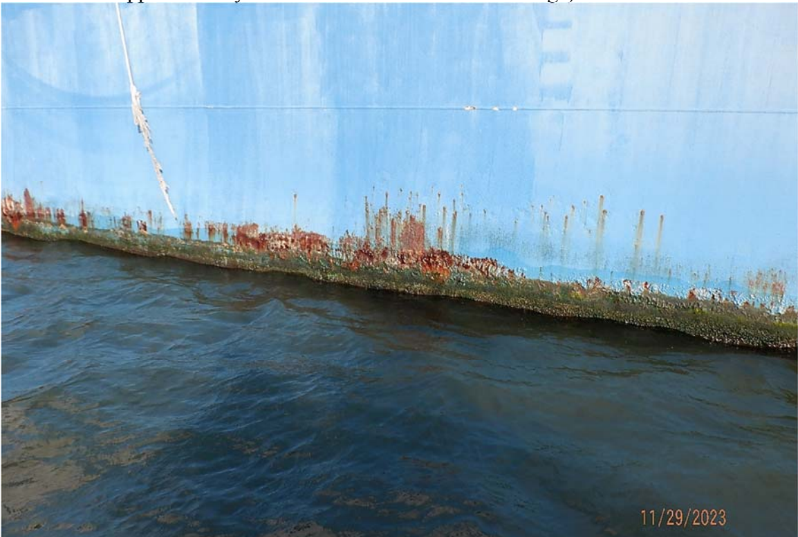
Photo 4.1-4: Minor coating loss and blistering with corrosion at the waterline along the south side of the barge.
