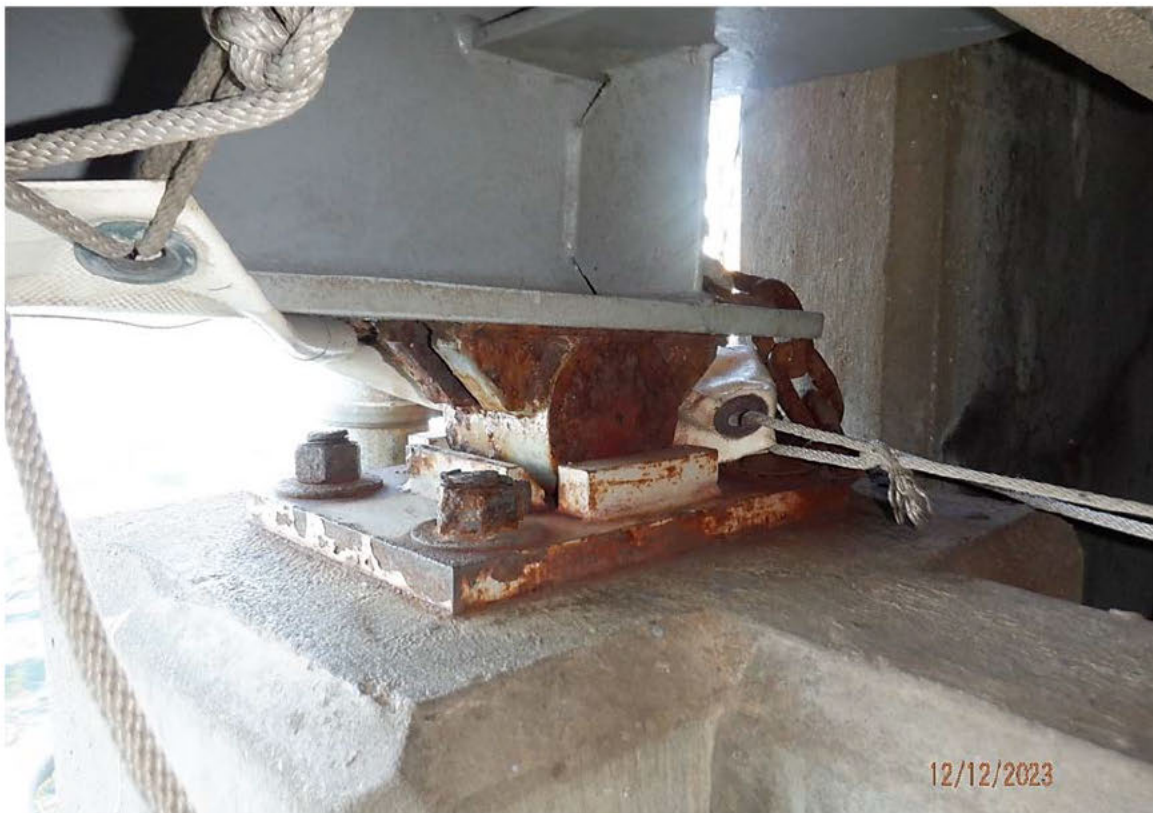
Photo 3.6-4: Condition of northwest rocker bearing at Pedestrian Gangway A. Assembly exhibits minor corrosion of the rocker bearing, bearing plate, and restraining safety chain. The anchor bolt nuts exhibit moderate to advanced corrosion.
