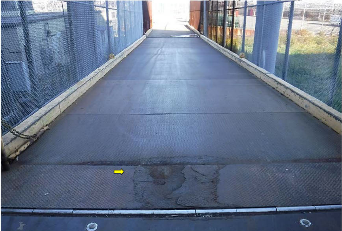
Photo 3.9-7: Overall view of the Cargo Gangway deck, curb, and security fence. Note the wear and corrosion on the transition plate.
