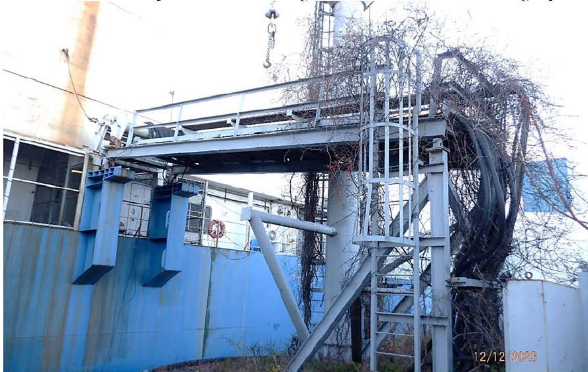
Photo 3.11-1: Overall view of the Electrical Gangway.
