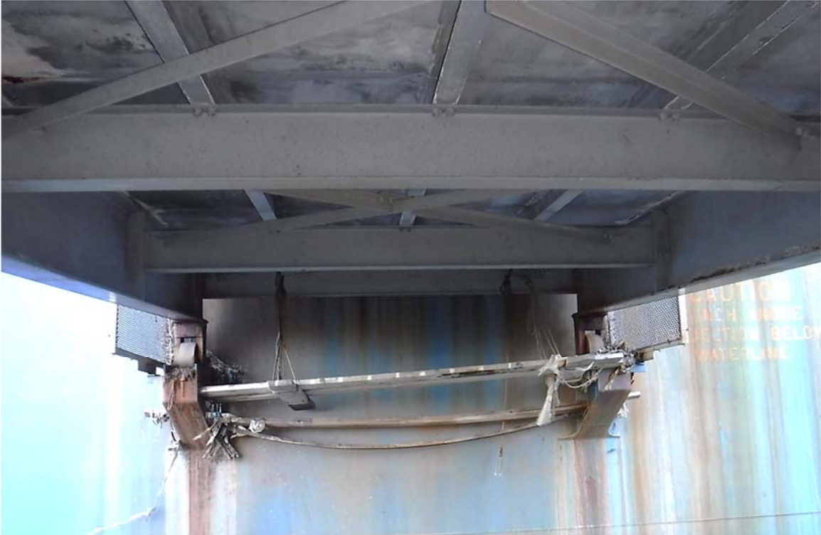
Photo 3.9-3: Overall view of the roller bearings at the Cargo Gangway. Note the debris interfering with the bearings.
