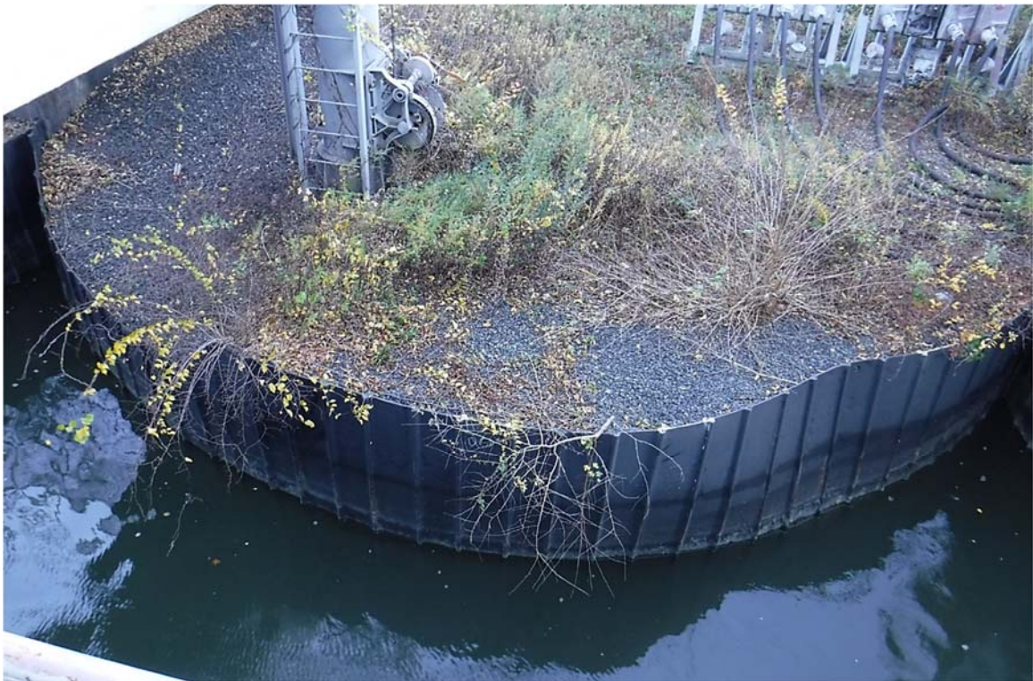
Photo 3.1-12: East side of Cell 3 is deformed, likely due to barge impact during installation.
