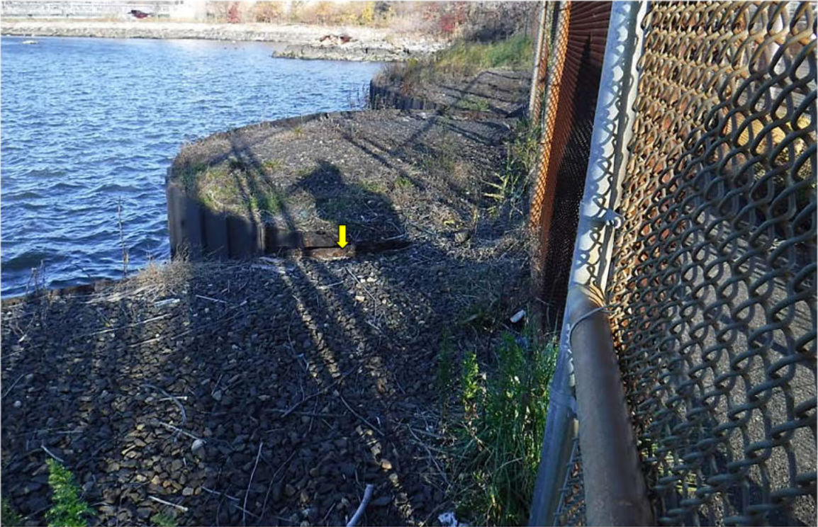
Photo 3.1-9: Subsidence at the north side of Cell 21 at approximately Sta. 1+22.
