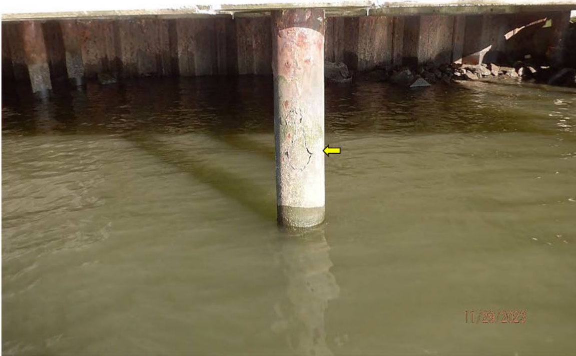
Photo 3.3-3: Typical minor coating loss in the tidal zone.
