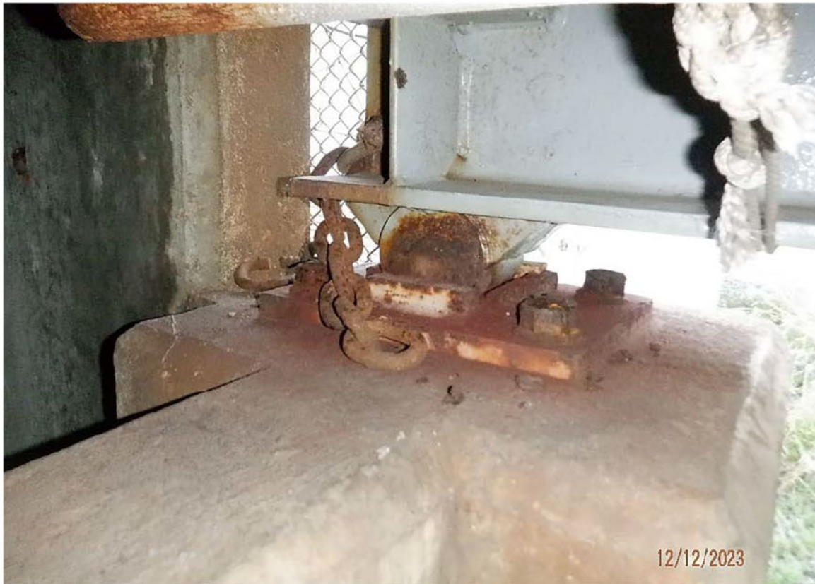
Photo 3.8-3: Example of typical anchor bolt and nut corrosion at the rocker bearings. Also note the broken or cut safety chain link at the northeast bearing.
