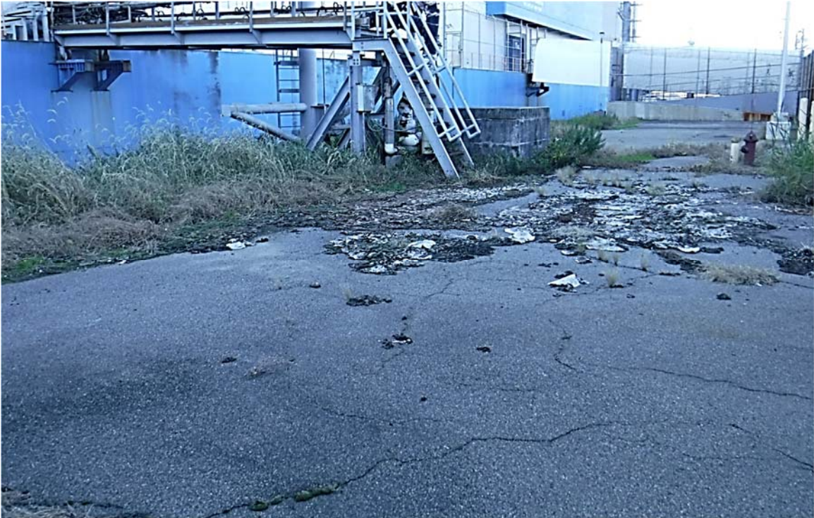
Photo 3.1-13: General view of the topside looking west of Cell 4. Note the remnant sanitary waste. The asphalt pavement is generally worn, uneven and contains many cracks. Also note the heavy overgrowth.
