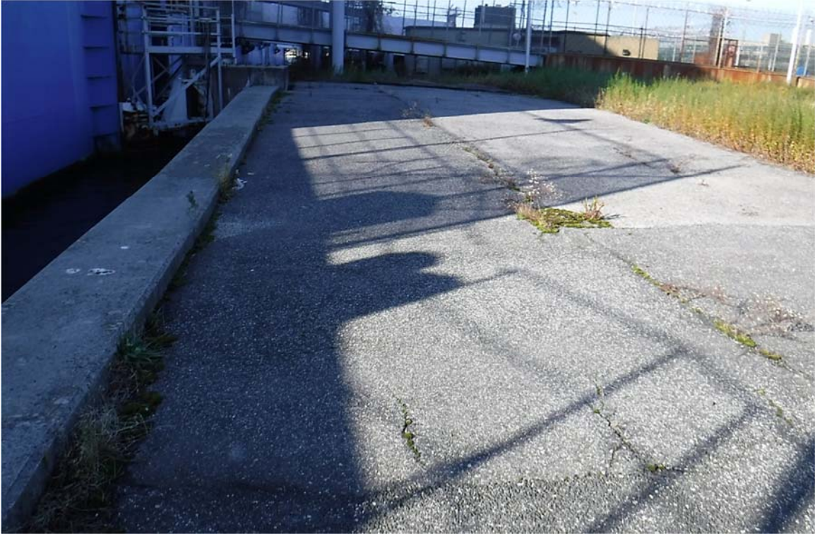
Photo 3.3-8: Overall view of the topside looking west. The pavement contains multiple cracks, excessive weathering, and the surface is uneven.
