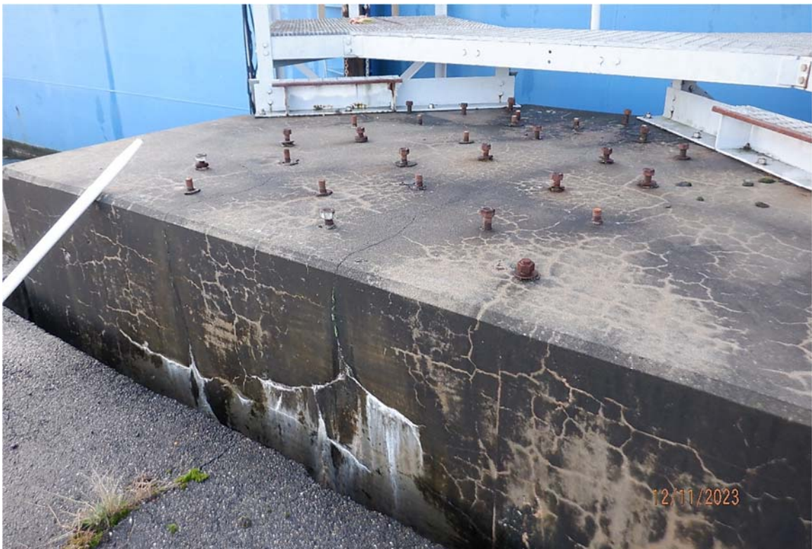
Photo 3.5-5: General view of cracks with efflorescence on the top face of the cap varying in width from general hairline map cracks up to 1/16".
