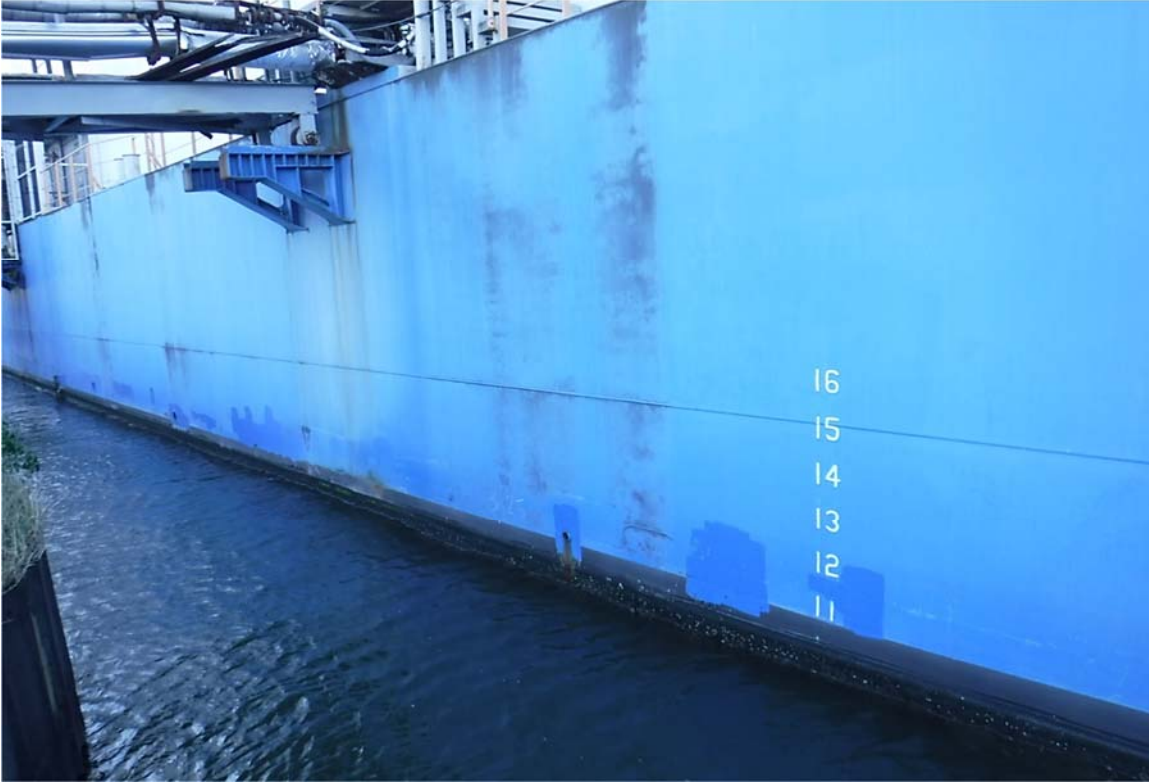
Photo 4.1-5: Barge markings indicate a draft of approximately 9'-8" below the waterline.
