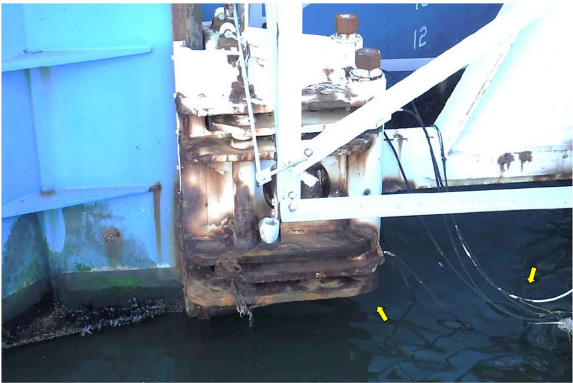
Photo 3.5-2: Closeup view of the east leg of the East Mooring Arm. Note the coating loss and corrosion of the assemblies immediately above the waterline. Also note the dangles grease hoses.
