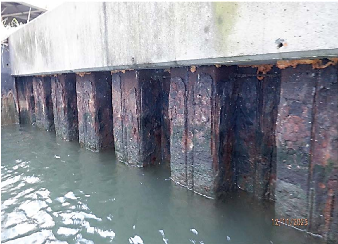
Photo 3.2-2: Closeup view of the moderate to advanced corrosion of the sheet piles in the splash zone above MHW.
