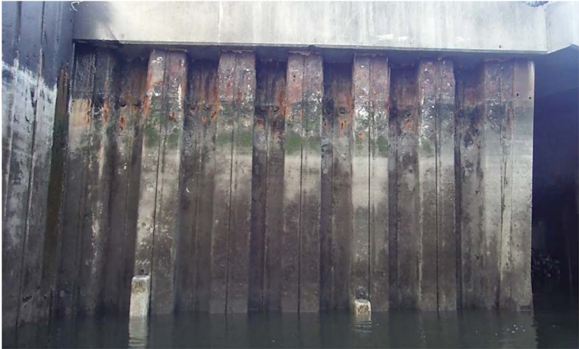
Photo 3.2-1: Overall view of the Transition Bulkhead sheet piles at MLW. Note two anodes protrude above the waterline.
