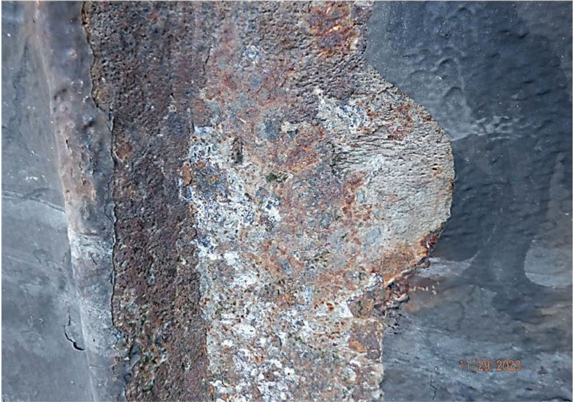
Photo 3.1-4: Closeup view of minor corrosion and pitting where the coating is failed.
