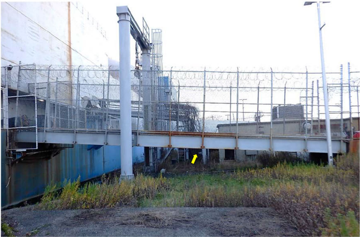
Photo 3.9-6: Overall east elevation view of the Cargo Gangway and support frame. Note the minor surface corrosion on the security fence posts along the girder.
