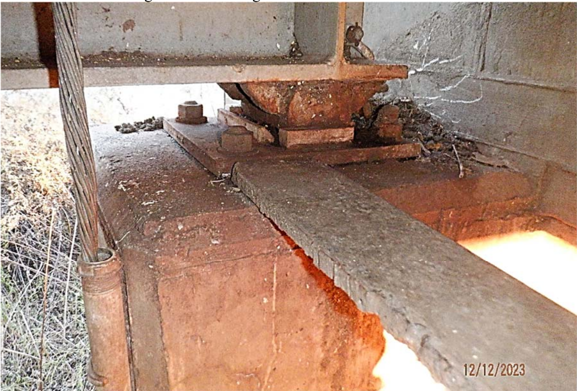
Photo 3.9-4: Debris accumulation and typical anchor nut corrosion as shown at the northwest rocker bearing.
