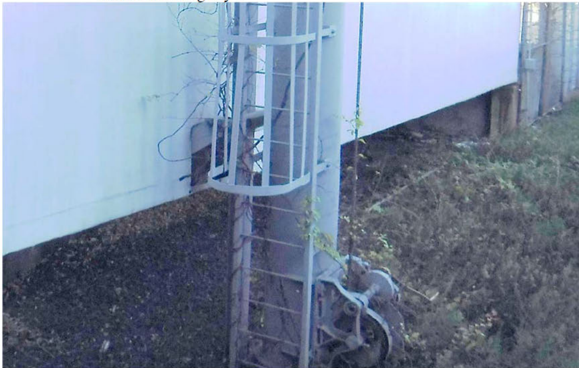
Photo 3.8-6: Moderate to heavy vegetation and vines growing on the support gangway cage ladder, mast, and winch restricting access and operation.
