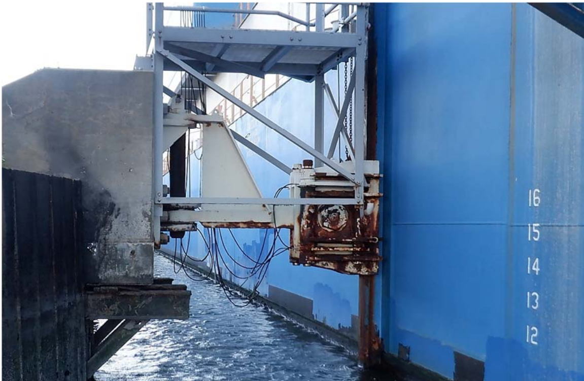
Photo 3.4-1: West elevation view of the single-leg mooring arm assembly. Note the coating loss and corrosion on the gripper clamps, leg, and T-guides.
