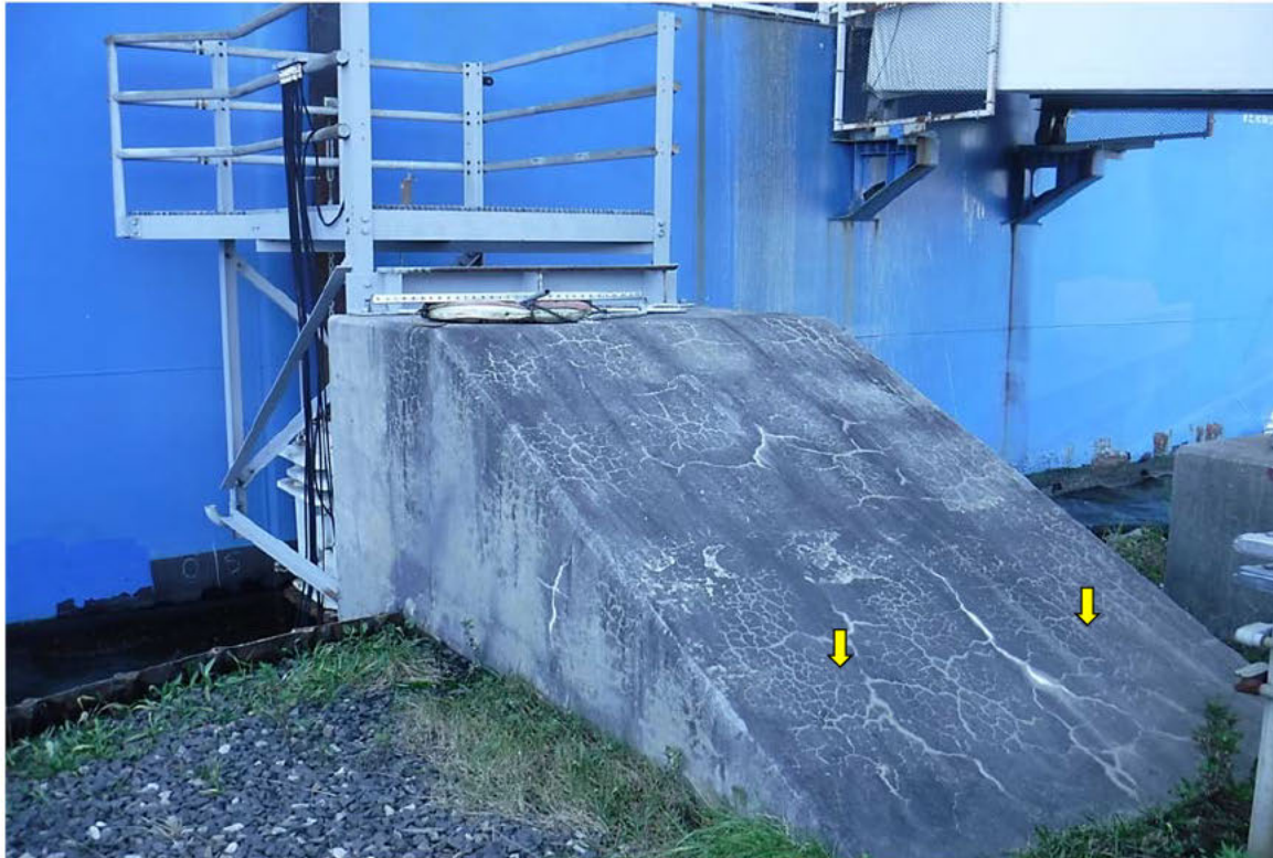
Photo 3.4-3: Overall view of the concrete support cap at the West Mooring Arm. Hollow sounding concrete exists where indicated by the yellow arrow.
