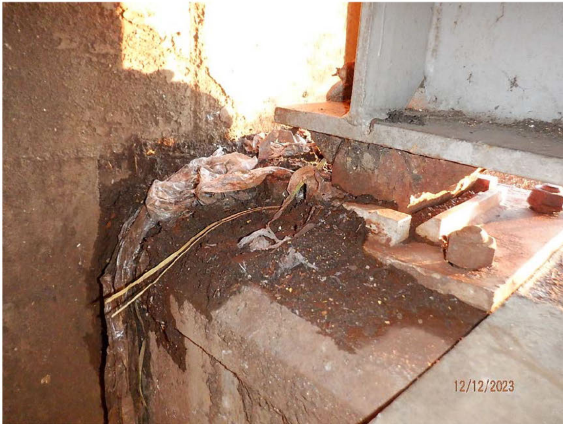
Photo 3.9-5: Debris accumulation at the northeast rocker bearing. Note the anchor nuts are not in contact with the bearing plate.
