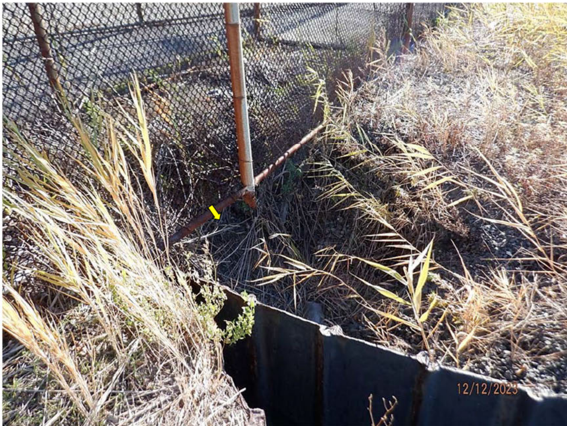
Photo 3.1-8: Sinkhole at the north side of Cell 24, approximately Sta. 0+40.
