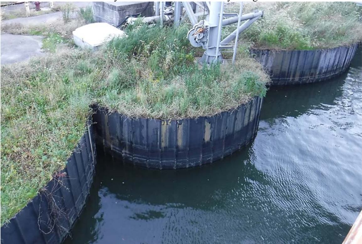
Photo 3.1-14: Typical excessive vegetation and overgrowth as shown at Cell 6.
