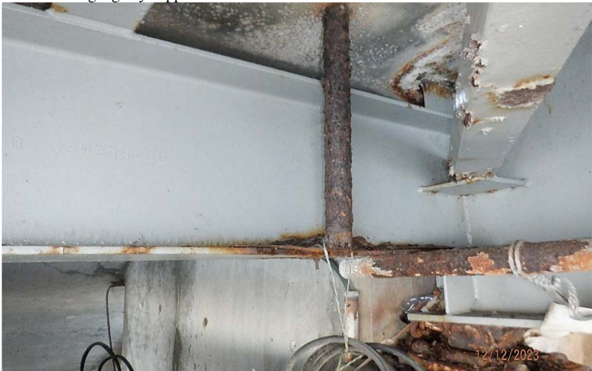
Photo 3.6-2: The bottom flange of the northernmost floor beam on its east side contains moderate corrosion and delamination. Also note the coating loss on the cross-bracing.
