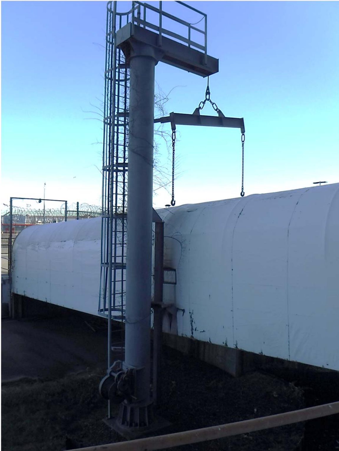
Photo 3.7-8: Overall elevational view of the gangway support frame at the Middle Pedestrian Gangway B. Note the vegetation growth along the steel cage ladder and mast. Some growth exists on the manual winch system.
