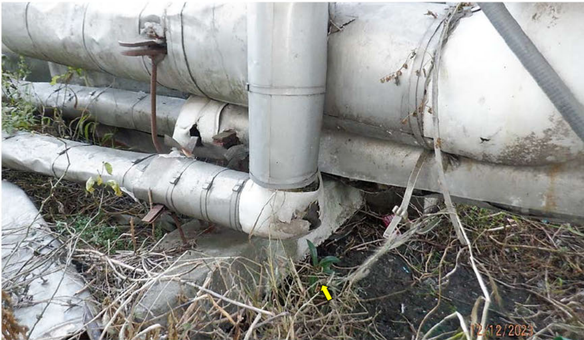
Photo 3.10-6: Example of impacted insulated utility lines at the Plumbing Gangway.
