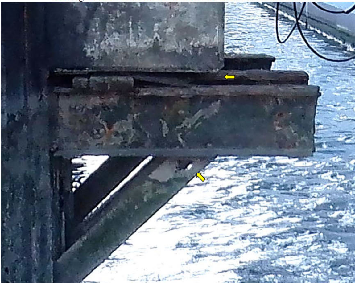
Photo 3.4-5: Closeup view of the corrosion hole in the western knee brace. Also note the gap between the top of the bracket and the underside of the support cap.
