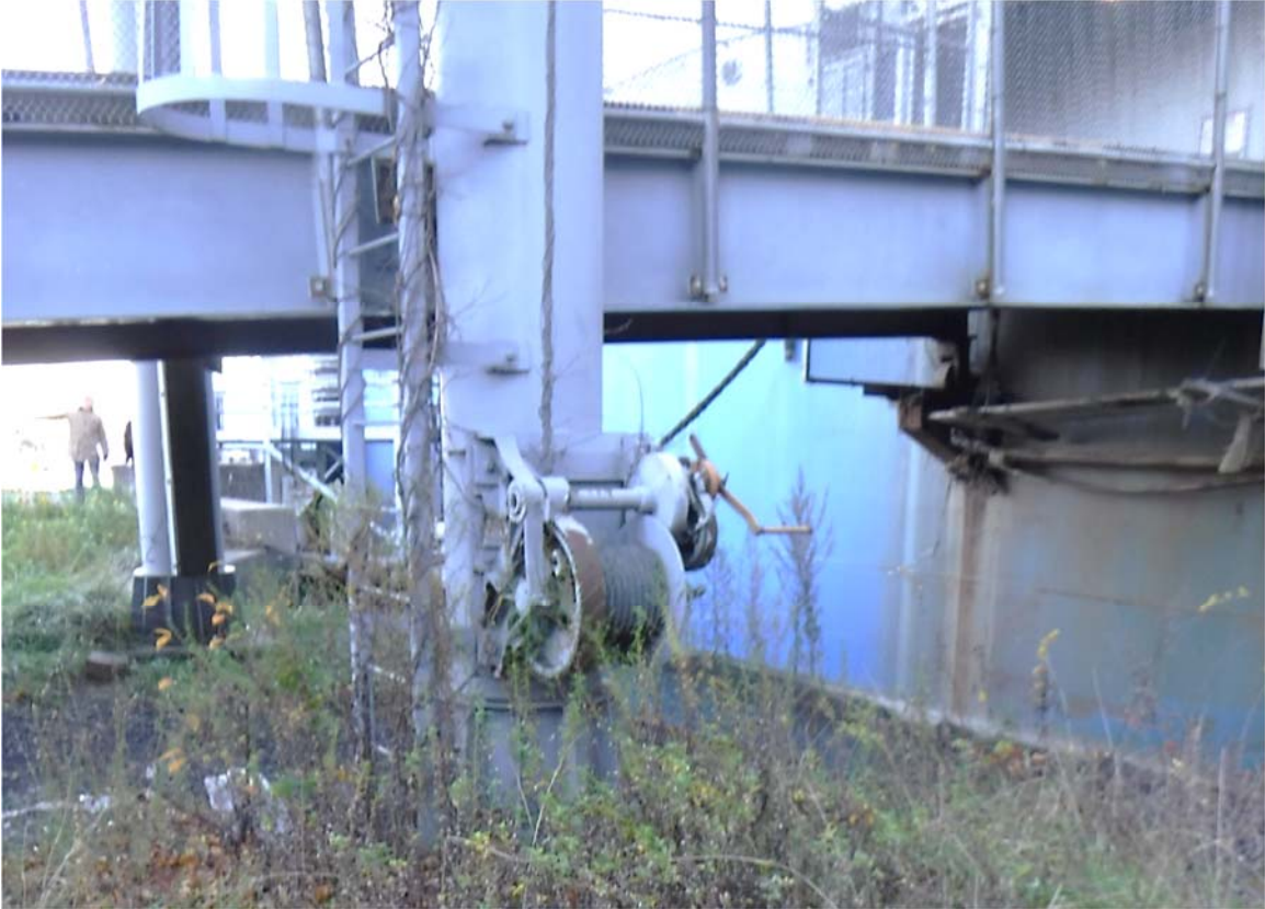
Photo 3.9-8: Moderate vegetation and vines growing on the support gangway cage ladder, mast, and winch restricting access and operation.
