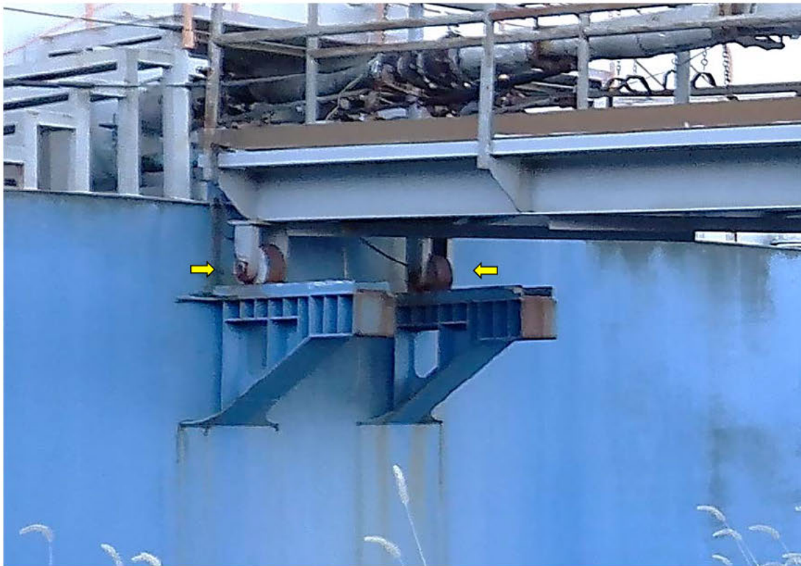
Photo 3.10-3: Enlarged view of the roller bearings at the Plumbing Gangway. Note the minor surface corrosion on the various surfaces.
