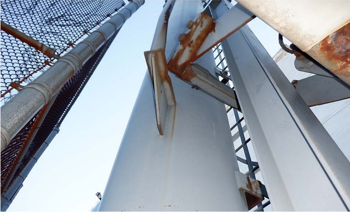
Photo 3.6-8: Guide bar framing interferes with a bracket appurtenance on the main mast. These elements conflict during low tide cycles, and the appurtenance is slightly deformed as a result.
