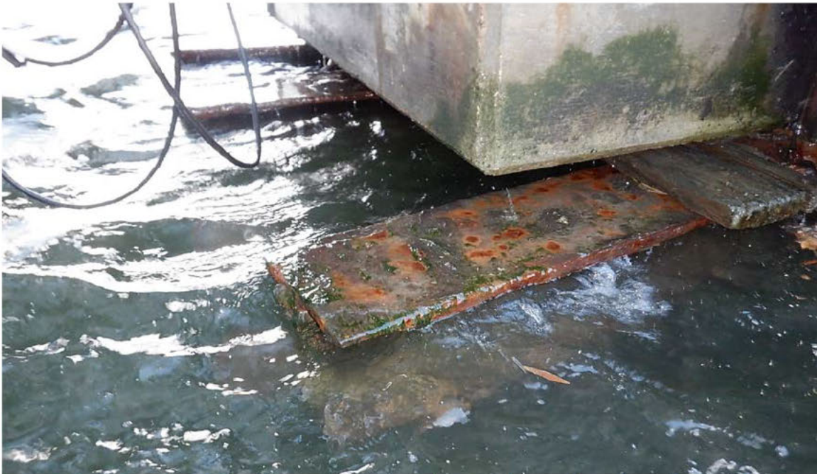
Photo 3.4-4: Coating loss with moderate corrosion on the steel bracket. Timber shims are missing between the steel bracket and the underside of the concrete.
