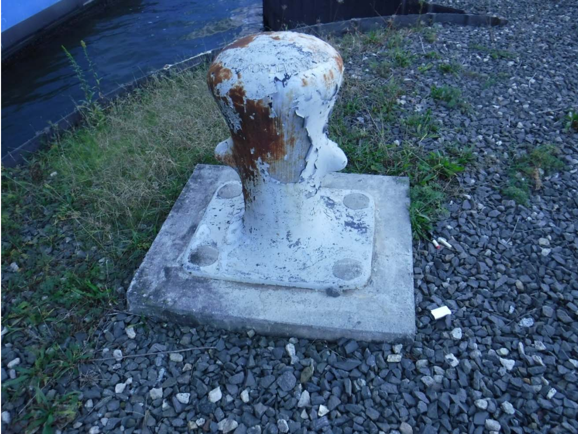
Photo 3.1-7: Bollard B-2 exhibits typical minor coating loss with surface rust. Note the anchor bolt pockets are filled.
