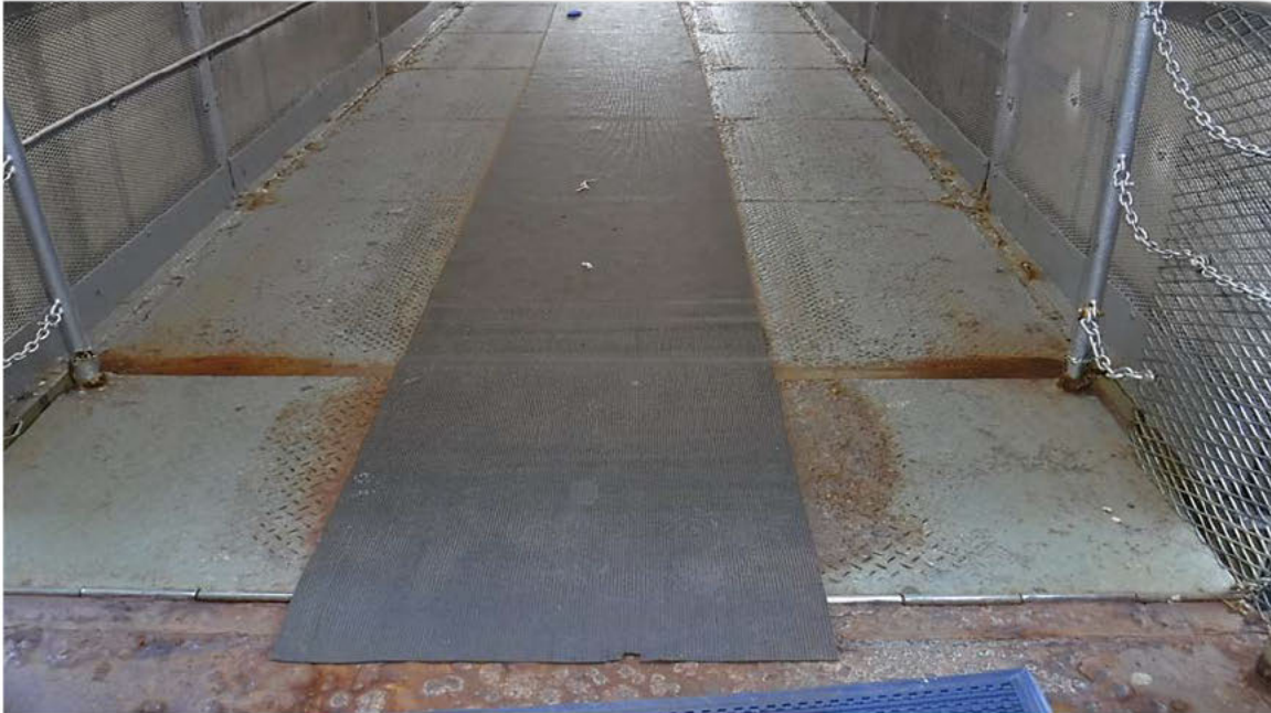
Photo 3.7-7: Interior view of the Middle Pedestrian Gangway B exhibiting wear with minor surface corrosion at various locations.
