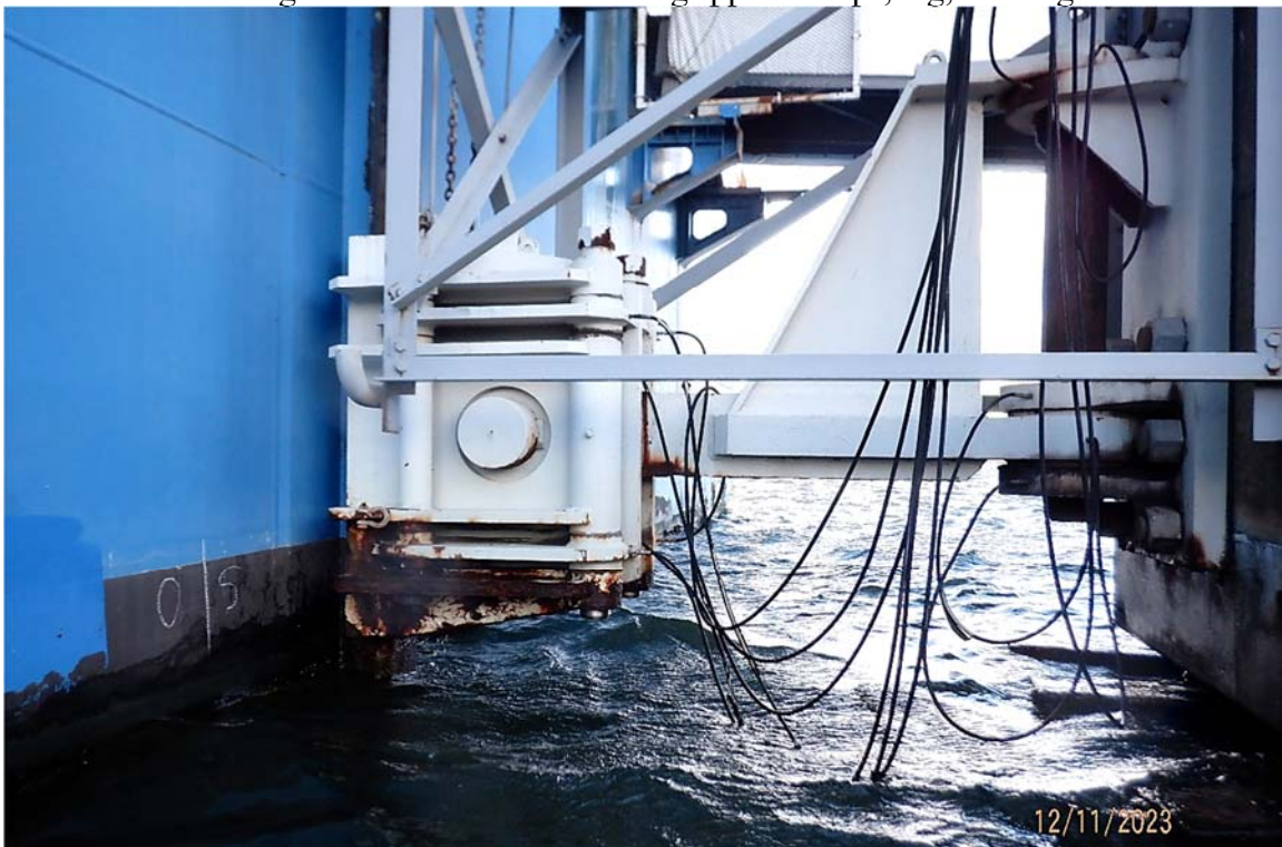
Photo 3.4-2: East elevation view of the single-leg mooring arm assembly. Note the coating loss and corrosion on the gripper clamps and anchor plate. Also note the grease fitting hoses hanging into the water.
