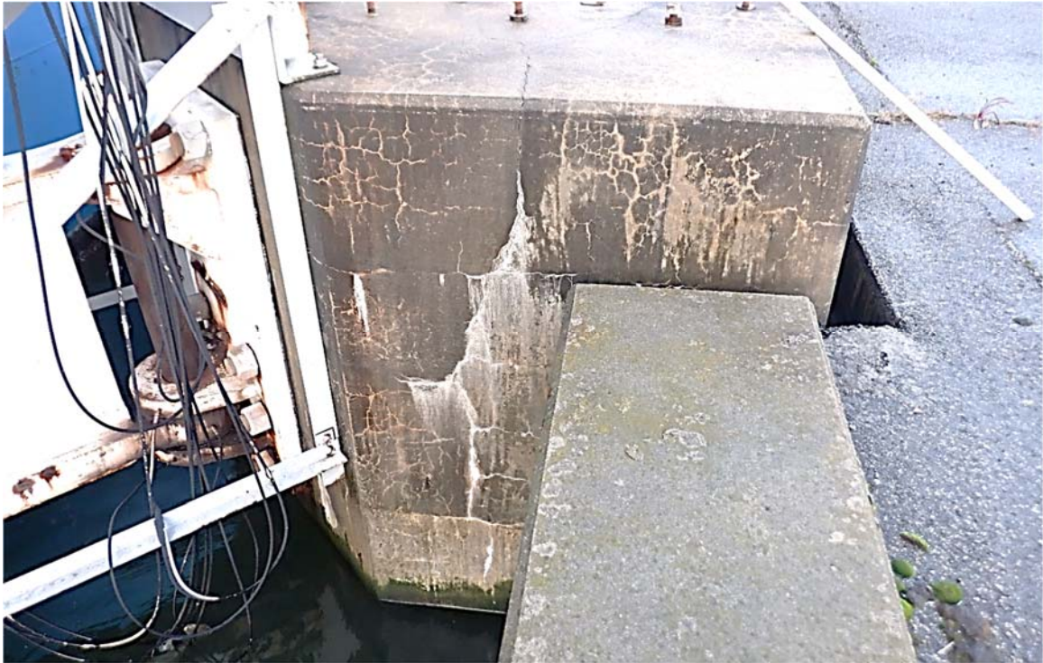
Photo 3.5-4: General view of cracks with efflorescence on the east face of the cap varying in width from general hairline map cracks up to 1/16".
