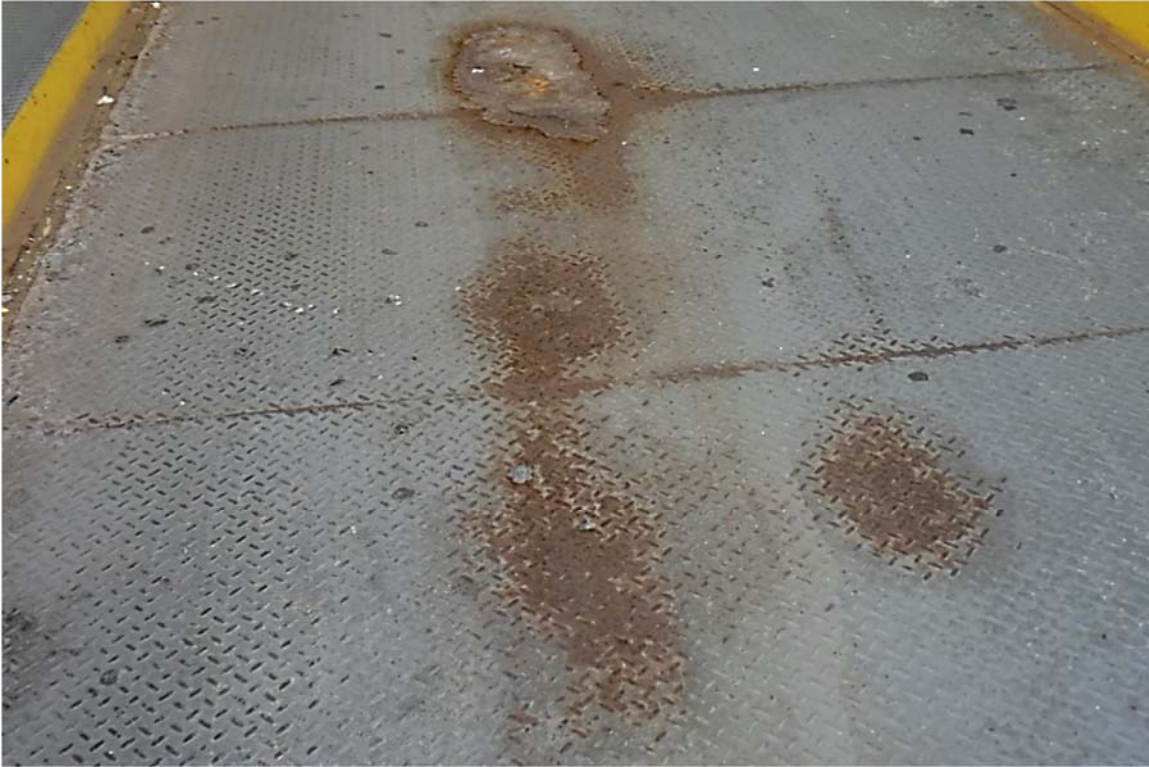
Photo 3.6-6: The steel diamond deck plate exhibits coating loss due to wear and abrasion at isolated locations. The steel exhibits minor to moderate surface rust.
