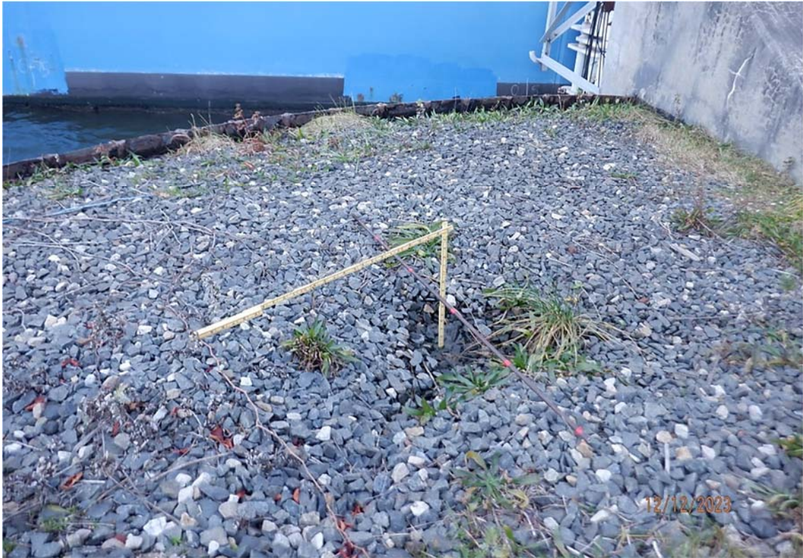
Photo 3.1-11: Minor sinkhole at Cell 15.
