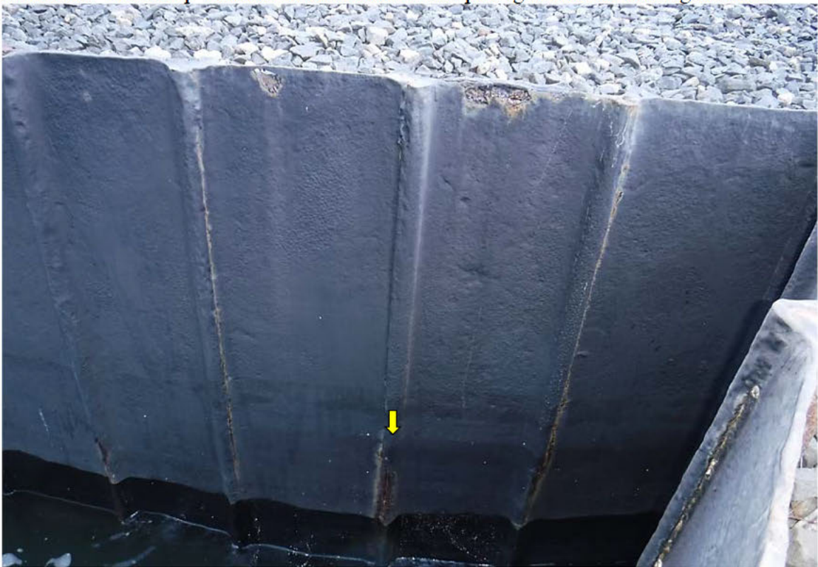
Photo 3.1-5: Typical coating failure on interlocking joints in the tidal zone. Note the previously pitted steel below the coating.
