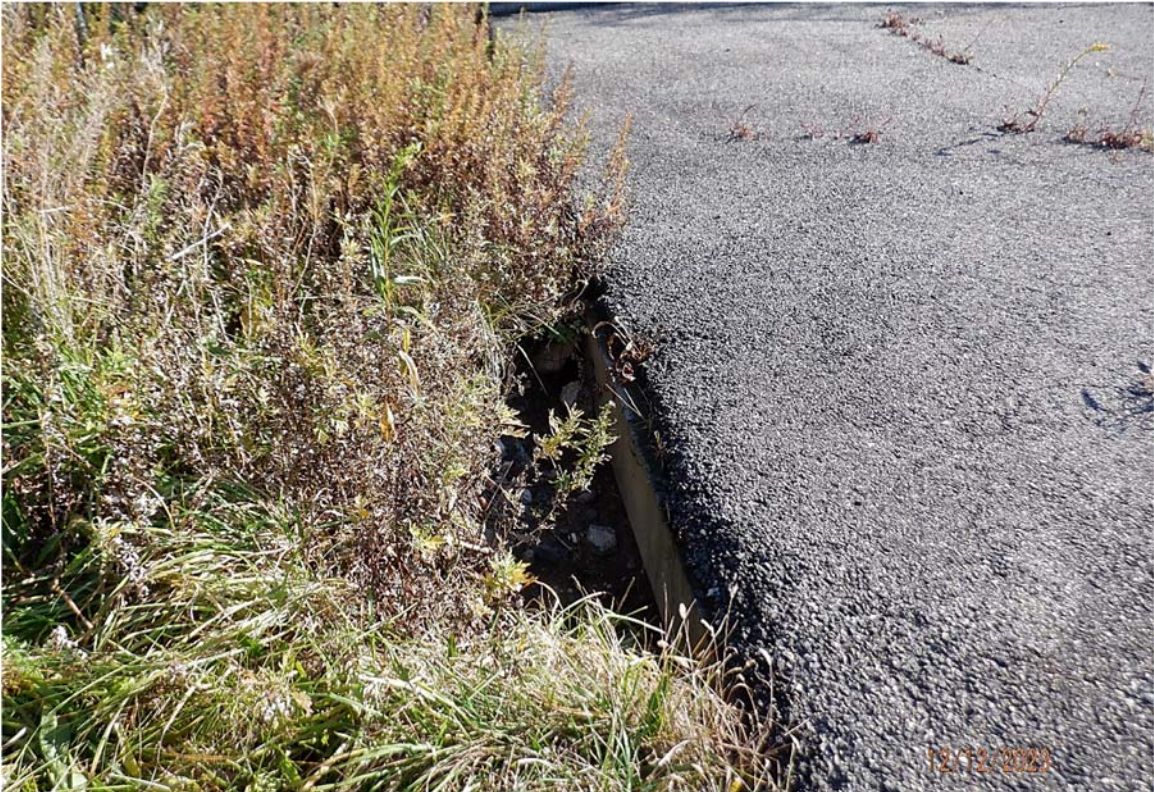
Photo 3.3-9: Sinkhole between Bents 1 and 3, approximately 18 in. deep.
