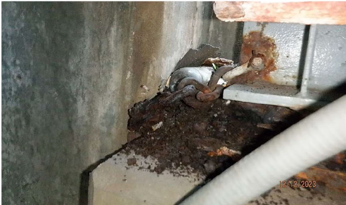
Photo 3.7-4: Closeup view of the northeast rocker bearing containing excessive debris accumulations at the Middle Gangway B.
