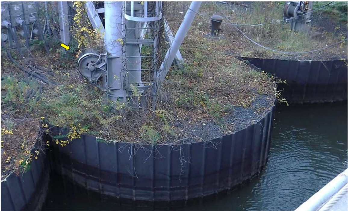
Photo 3.11-4: Excessive growth in the winch mechanisms at the Electrical Gangway.
