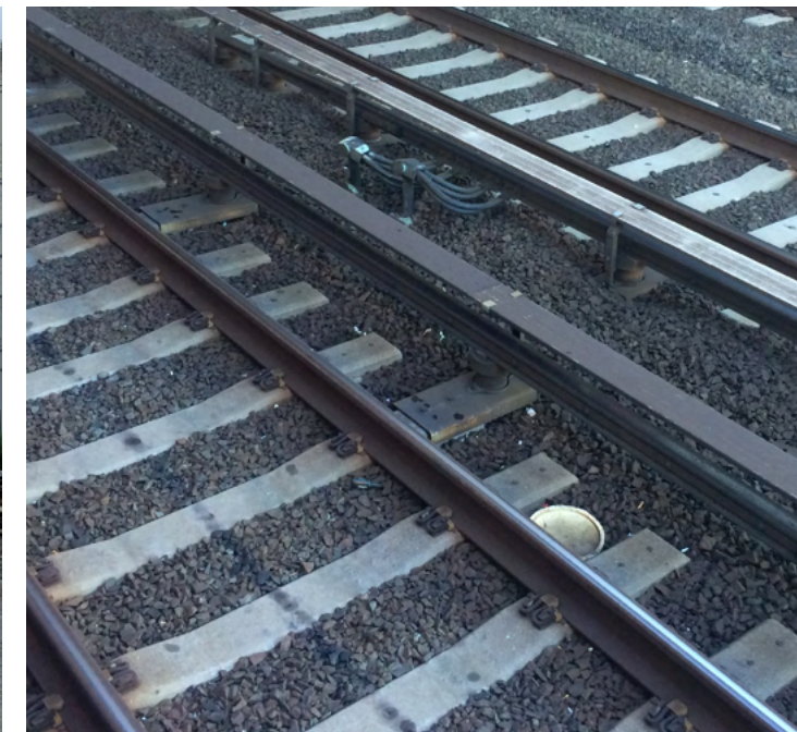
FIGURE 3.4: THIRD RAIL WITHIN SUNNYSIDE YARD
