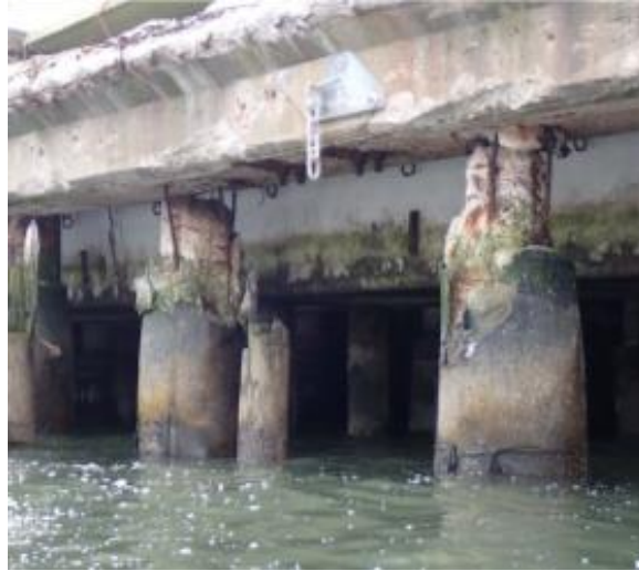
Need to repair our crumbling infrastructure and adapt to rising seas
