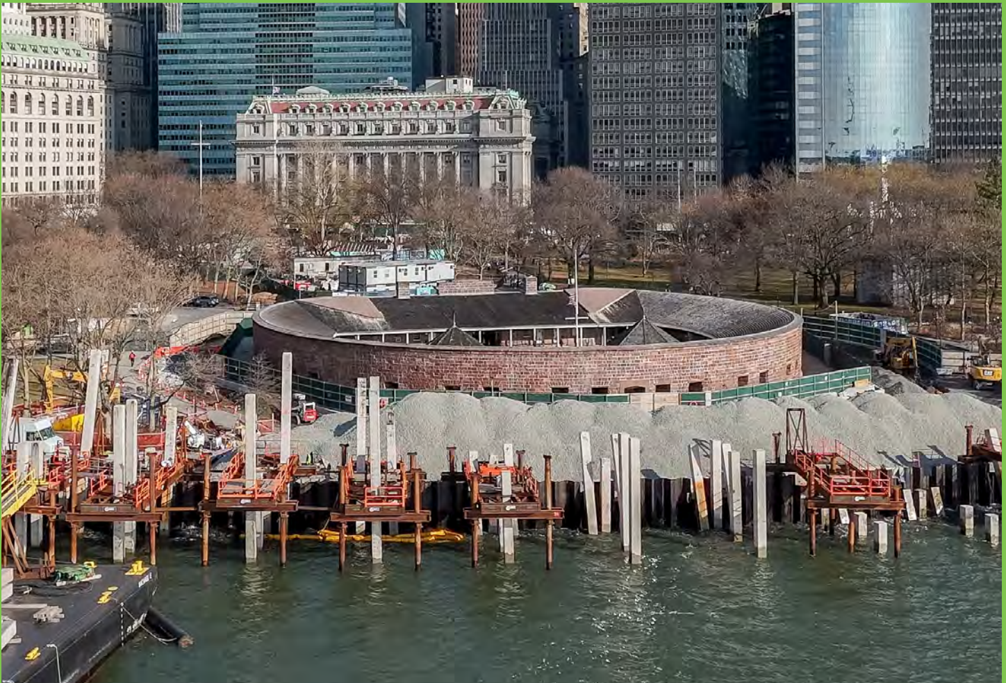
The Battery Coastal Resilience Project, a coastal protection initiative to reduce flood risk.
