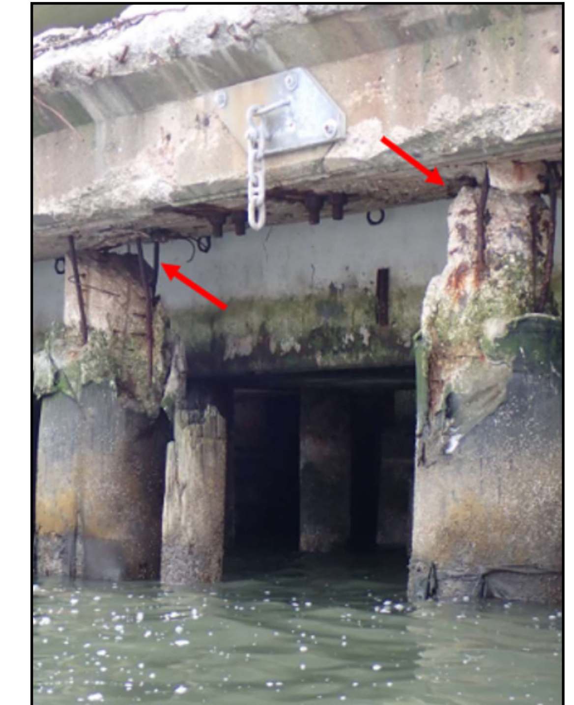
Deteriorated piles at BMT
