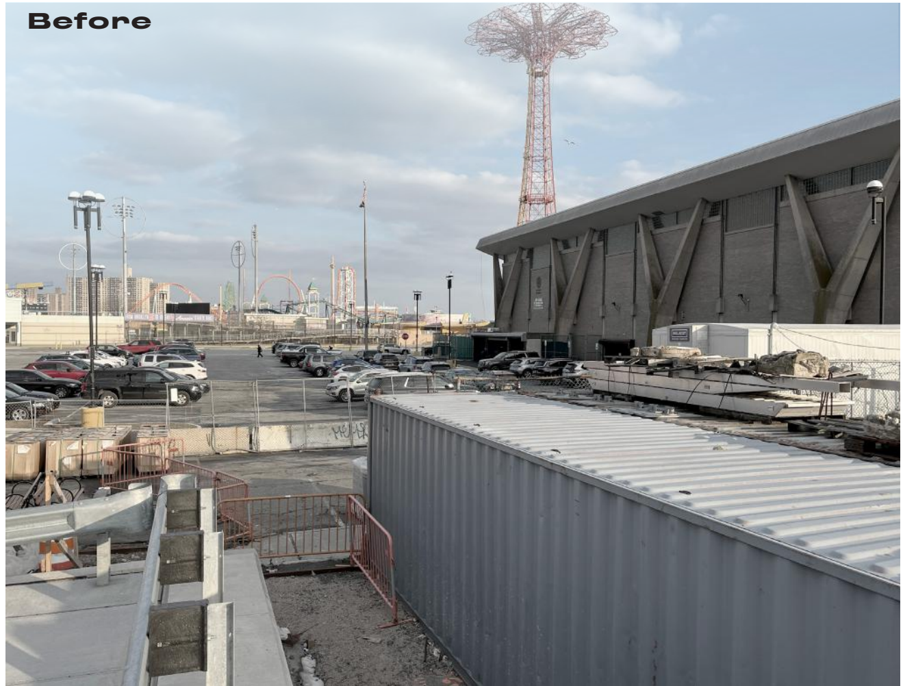
Parking lot and Ocean Way construction Existing condition (left, Source: NYCEDC) Future intersection of Ocean Way & West 20th St with renovated Abe Stark Sports Center and development on Parcels E & F. (right, Rendering by ONE Architecture & Urbanism)
