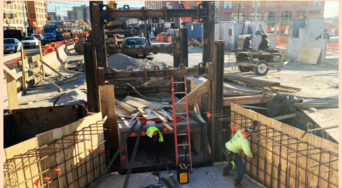
Construction of new sewers with Surf Vets Place in background (Source: NYCEDC).
