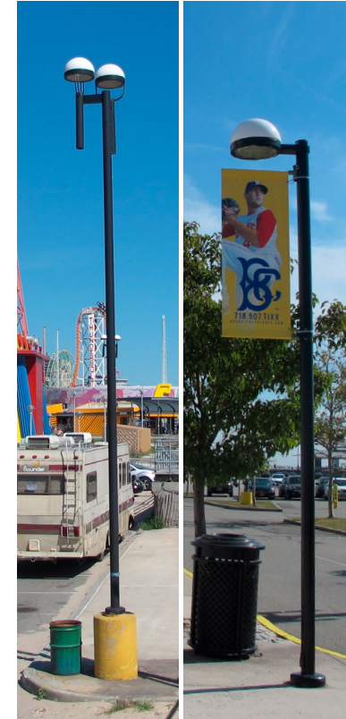
MCU Park parking lot and sidewalk lighting
