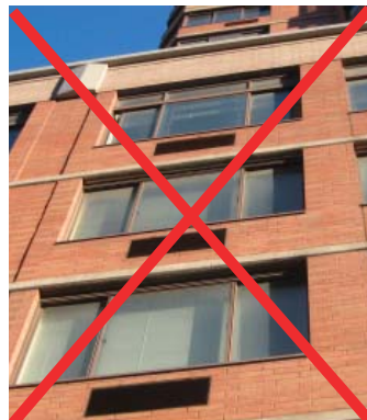
Avoid exposed slab edges, and punched A/C units
