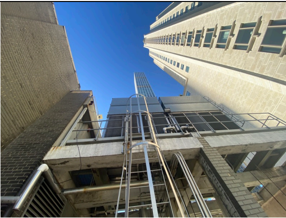
3. Rooftop Cooling Tower
