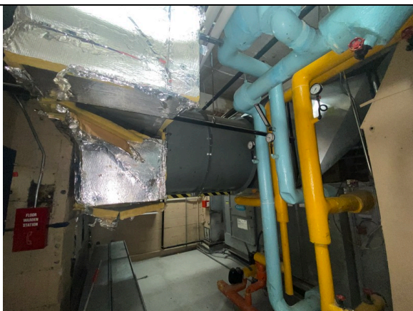
21. Mechanical Equipment for HVAC and Steam Systems (Located in a mechanical closet on each floor)
