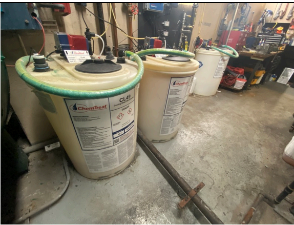
9. Microbiocide Drums for Cooling Tower
