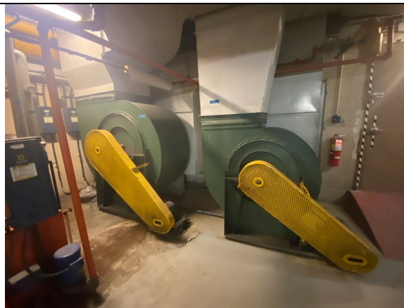
20. Mechanical Equipment for HVAC and Steam System
