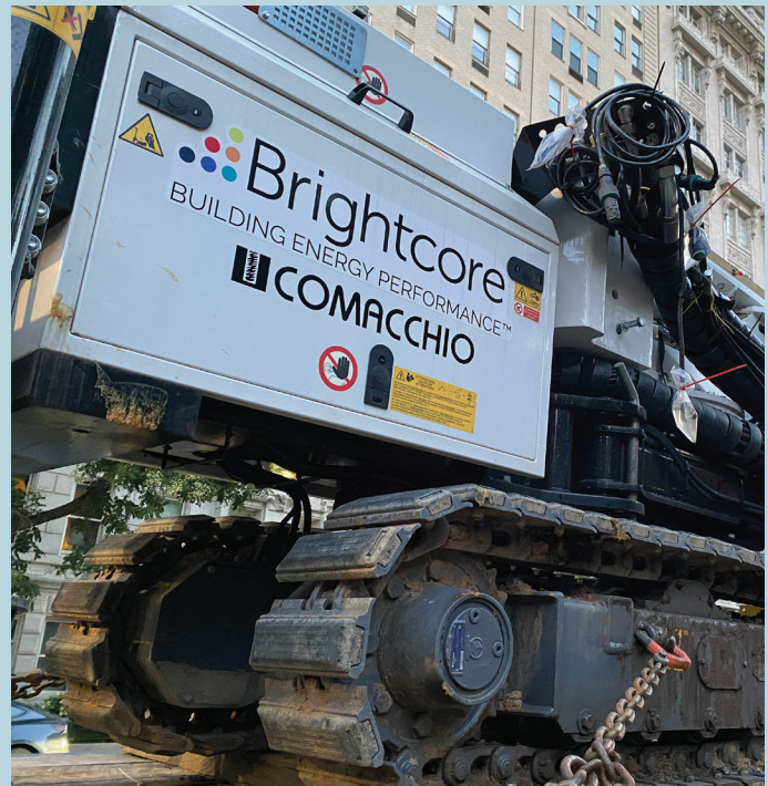
Brightcore Energy develops, implements, funds, and maintains end-to-end energy efficiency and renewable energy solutions. Source: Brightcore Energy
