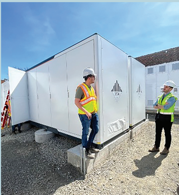
Microgrid Networks team testing new battery modules at Maspeth facility. Source: MGN
