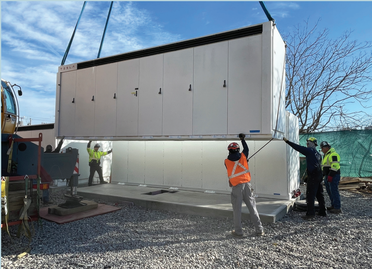
NineDot Energy installs a battery storage system in NYC. Source: NineDot Energy
