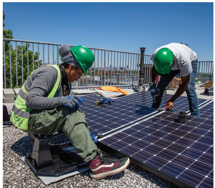
Solar power is installed at NYCHA buildings. Source: NYCHA
