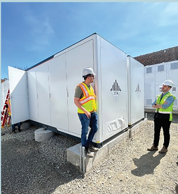
Microgrid Networks team testing new battery modules at Maspeth facility. Source: MGN
