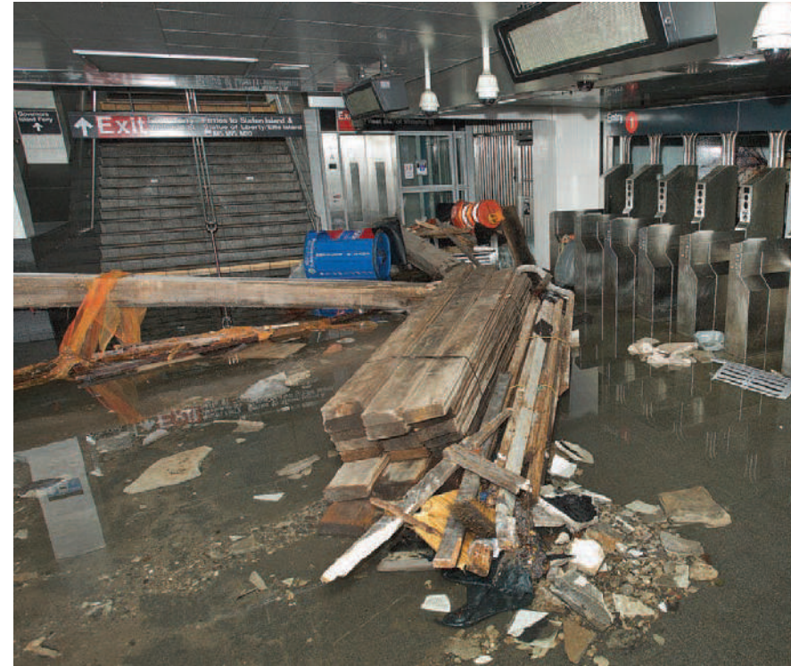
South Ferry Station in Lower Manhattan flooded to the mezzanine level after Hurricane Sandy (Photo Credit: MTA)
