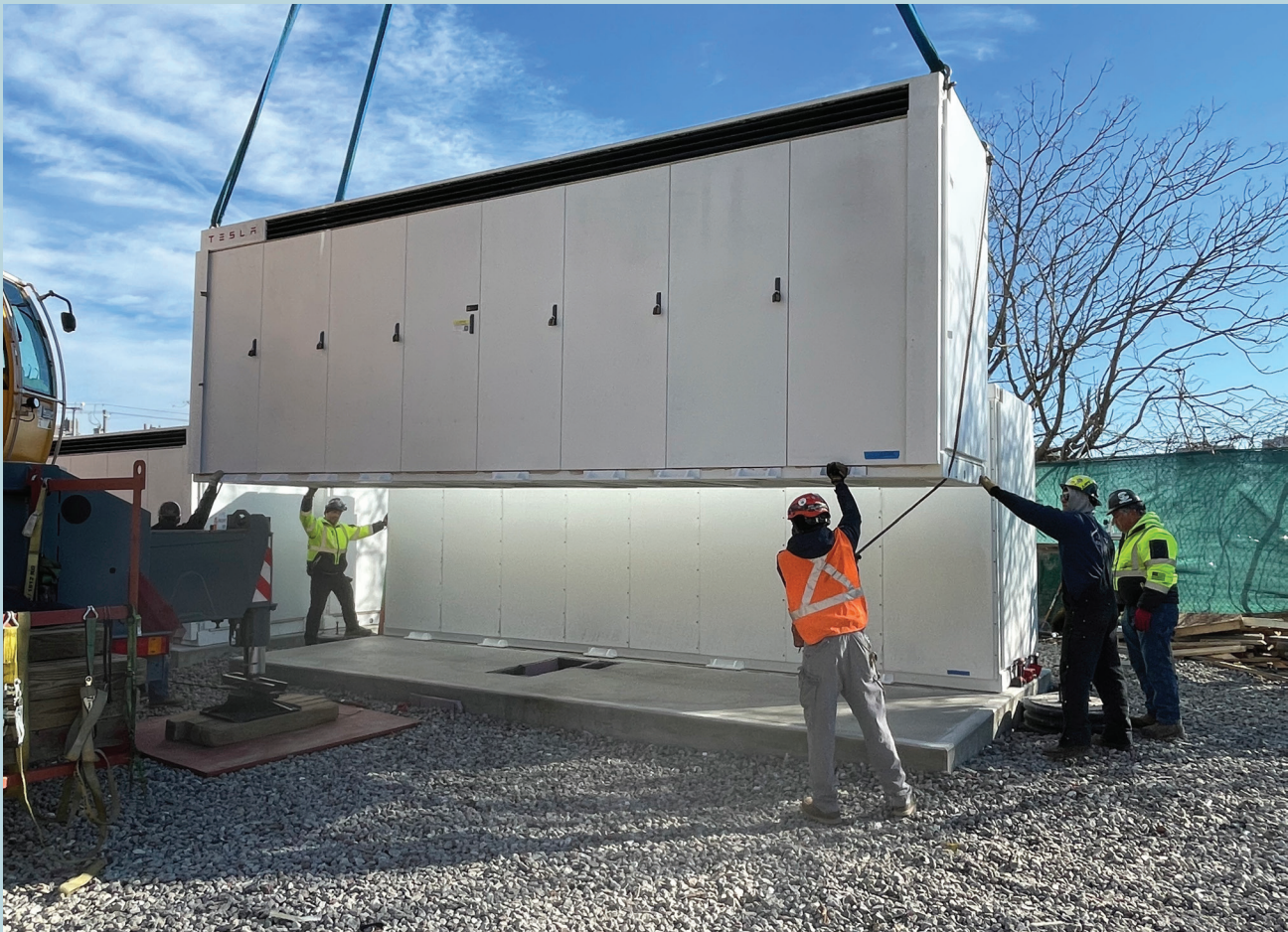
NineDot Energy installs a battery storage system in NYC. Source: NineDot Energy
