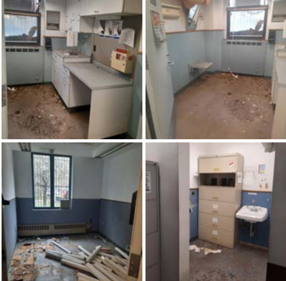
The facilities at 60 Madison Street need capital renovations and repairs before they can be reopened as a health center.
