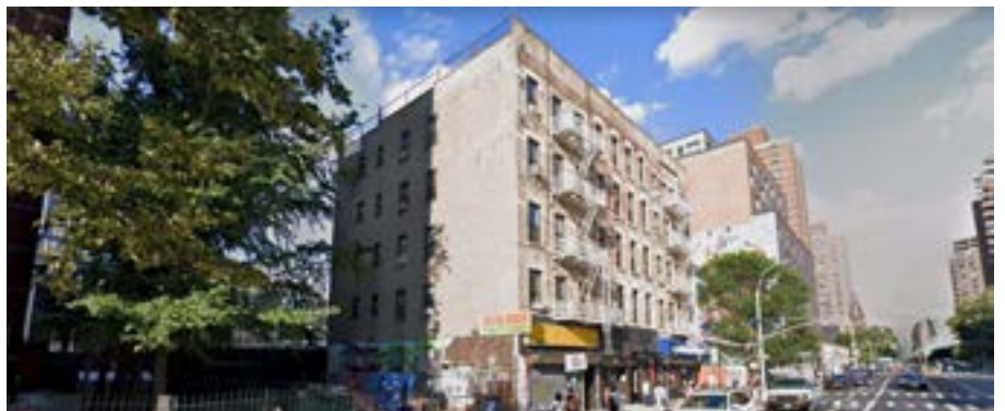
Screenshot of the existing wall at 384 Grand Street, image source: Google Maps.
