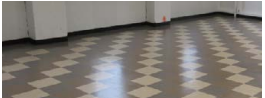
New tile flooring was added as part of structural repair work in the wake of Hurricane Sandy.
