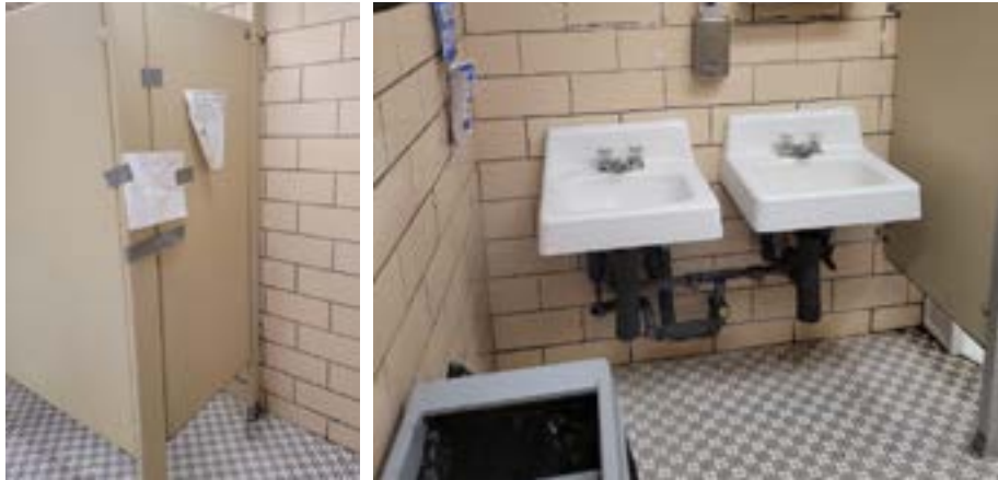
HMH's current restrooms are not ADA compliant.
