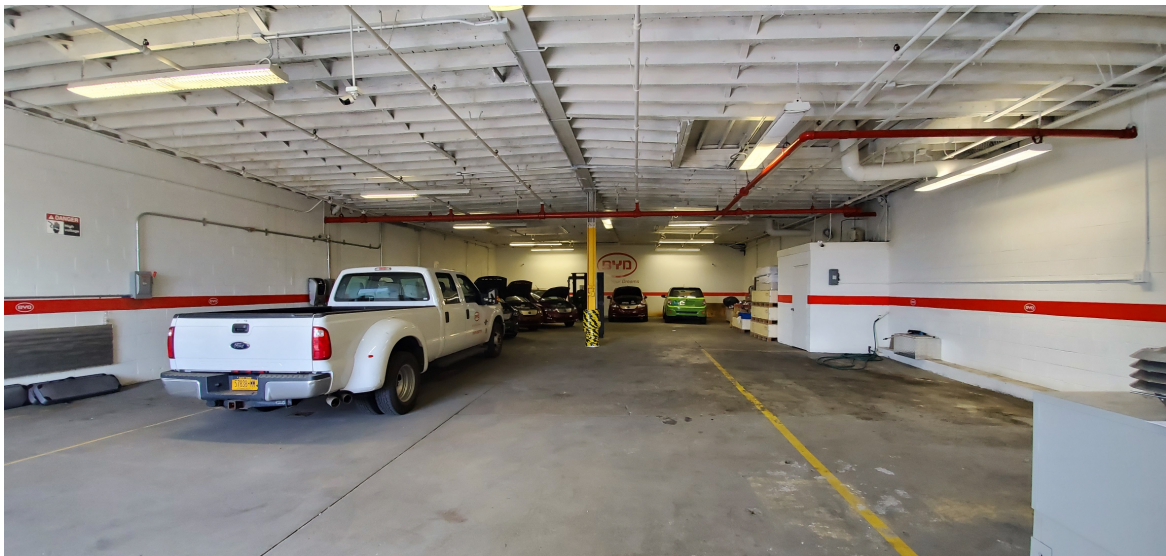
Ground Floor EV Charging Area
