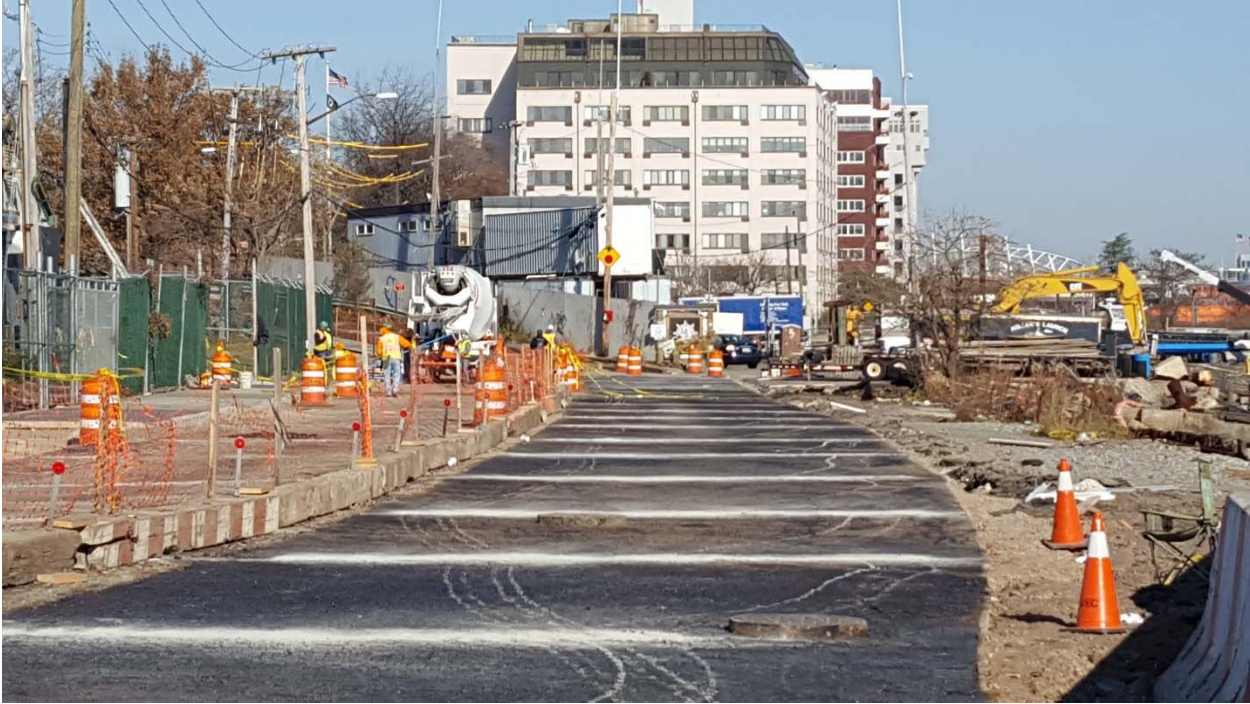
Start of Permanent Restoration of Front Street (looking north towards Hannah Street)
