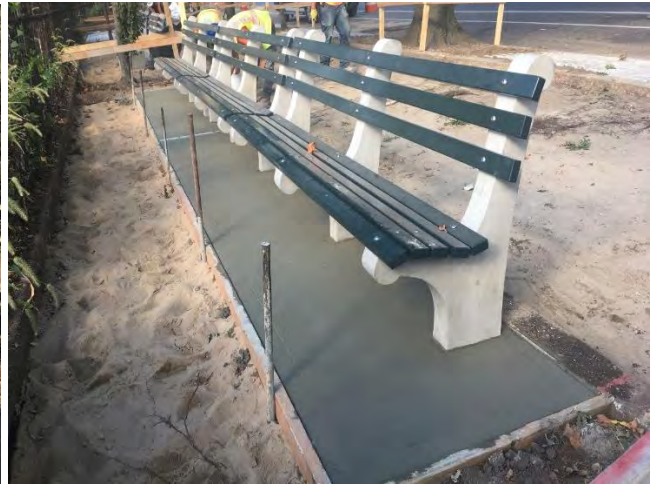
Installation of new Park Benches and Concrete Strip along Shore Road, adjacent to Shore Road Park
