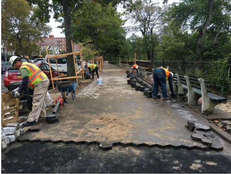
Installation of hexagon pavers along Shore Road, between 83 rd and 86 th Streets
